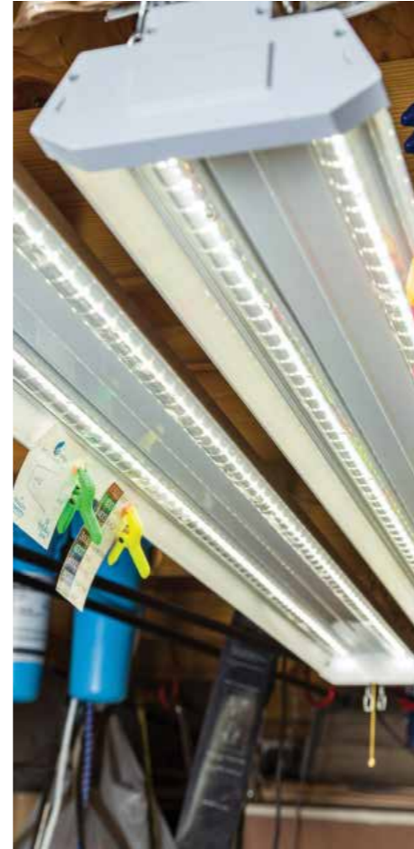
Get as much lighting as you can, located directly overhead along with any task lighting you might need
